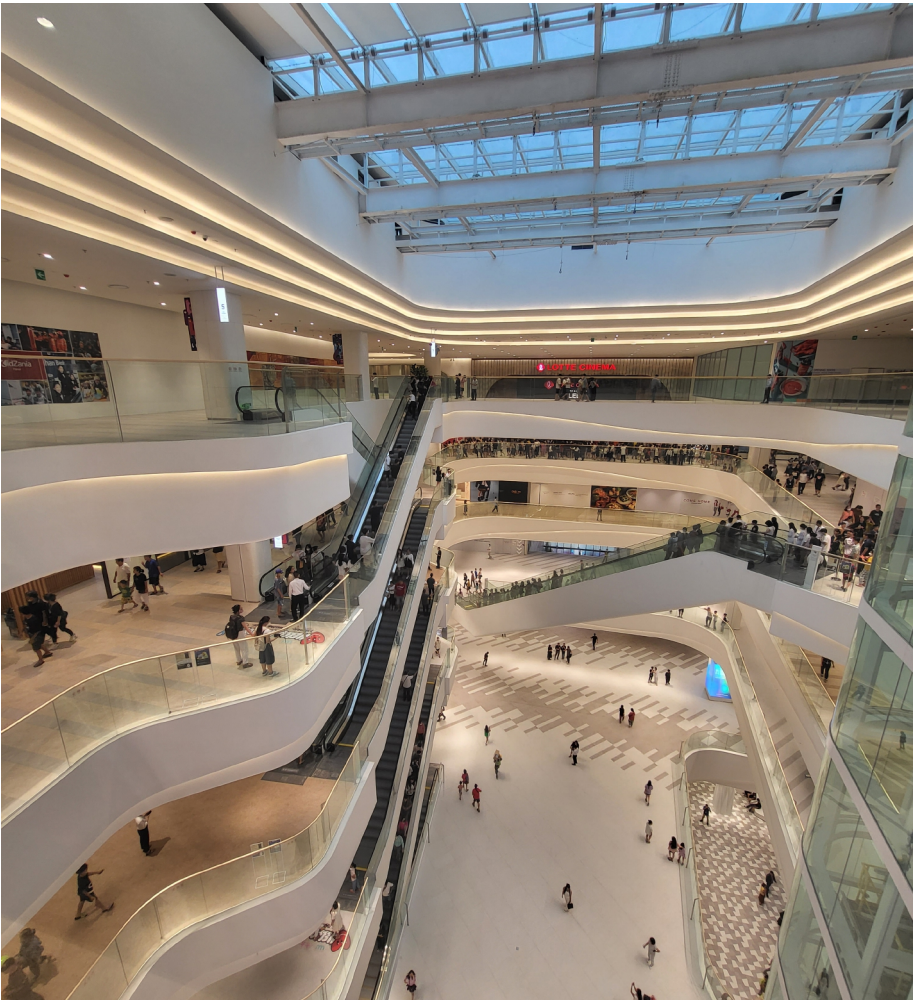
Wireless lighting control for a complete shopping mall: Tridonic supplied basicDIM Wireless passive module G2 application controllers and drivers for the various luminaires in the Lotte Mall in Hanoi, Vietnam. The application controllers can be managed wirelessly via an Android or iOS device and do not require a gateway.
