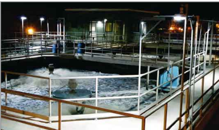
Figure 9: View of the plant with the final installation.
