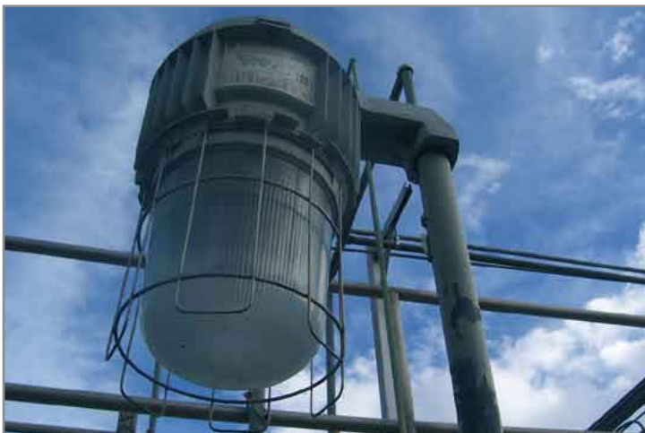
Figure 3: The existing type of lighting fixture used on the installation. This type of fixture is used extensively in the North American market and has been in production for many years.
